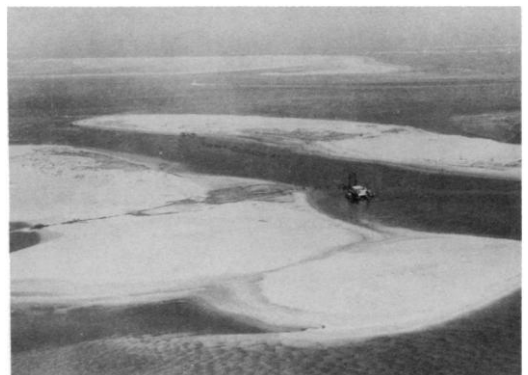
Figure 4. Hydraulic dredge working a channel in southeastern North Carolina, creating a new island. Photograph by James F. Parnell.
